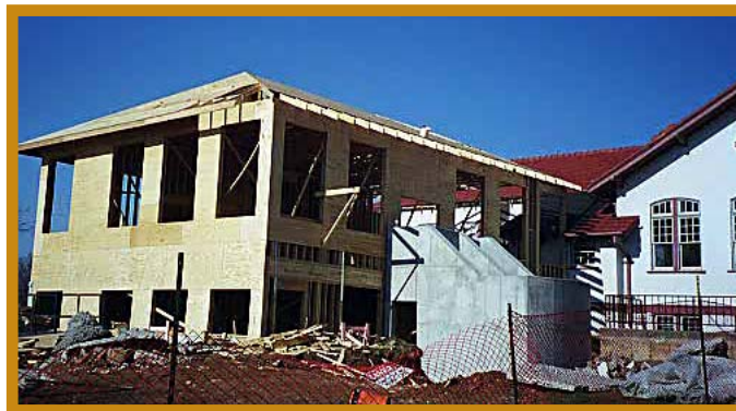
As construction progresses, the new addition prepares to meet the historic 1915 chapel.
