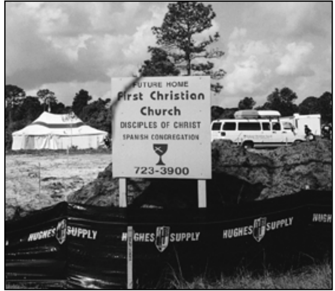
More than 100 volunteers from seven states have been in Florida to help construct a new building for Misión Cristiana de Palm Bay, a growing Disciples congregation outside of Melbourne. BCE approved loans totalling $300,000 for the project.
